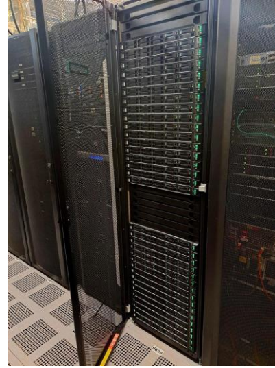
Datacenter FRMCS 5G Core
